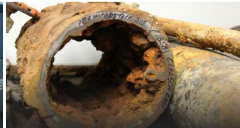
Decaying infrastructure assets
